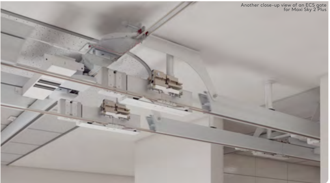
Close-up view of the ECS gate system
